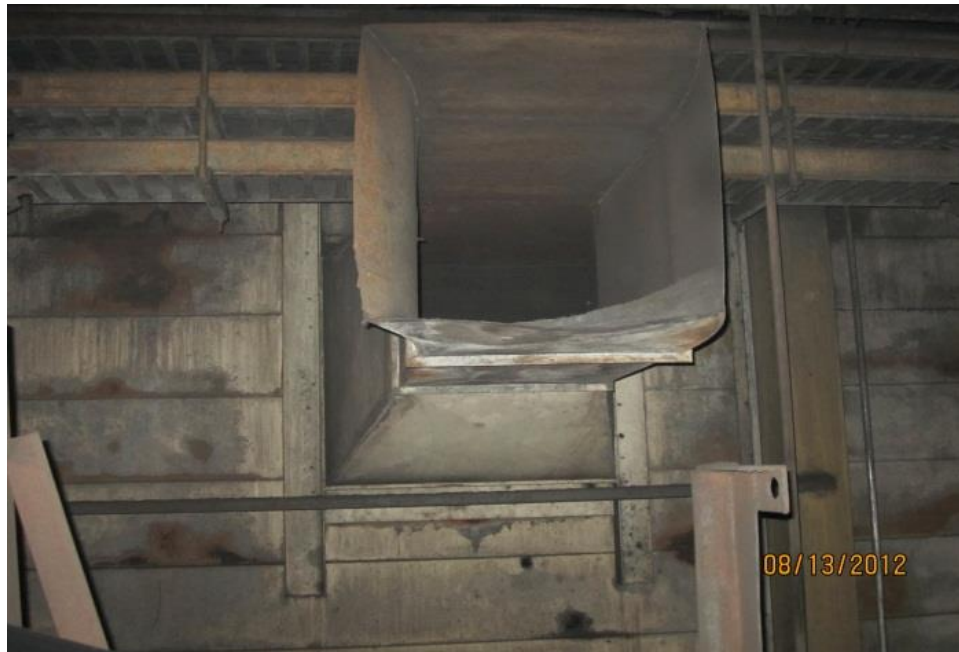
Picture 13: Duct work from an abandoned dust collector system as observed at CUF on August 13, 2012, in the Unit 1 South Bunker room (BC-25).
