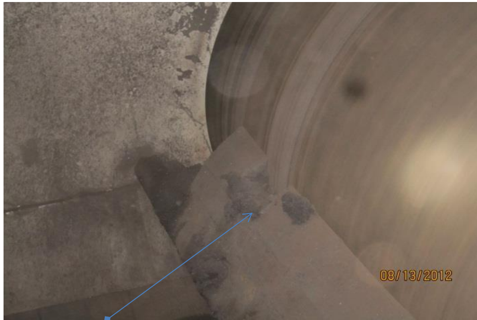
Picture 10: A gouge in a belt cleaner causing coal dust leaks as observed at CUF on August 13, 2012, along BC-16.
