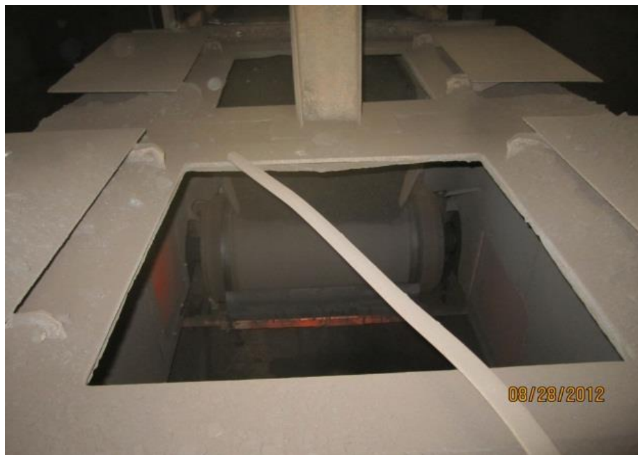
Picture 15: Open coal chute doors above the feeder platform as observed at PAF on August 28, 2012. We also observed open and deteriorating chute doors at head pulleys, tail pulleys, transfer points, and feeders at BRF and CUF. Open chute doors allow dust to be expelled into the surrounding area, adding to housekeeping efforts and increasing the hazard of coal dust explosions.
