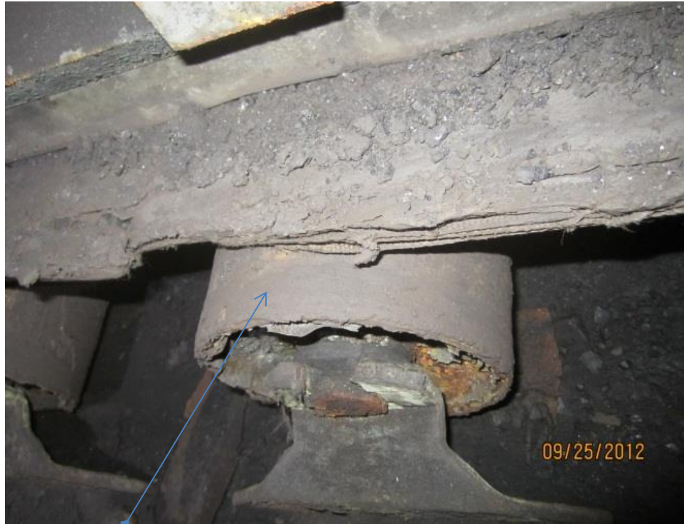
Picture 8: A worn belt due to misalignment causing coal dust leaks as observed at BRF on September 25, 2012, along Belt Feeder 2.
