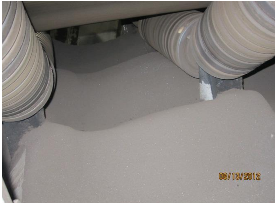
Picture 16: Coal and dust accumulations on idlers at a tail pulley as observed at CUF on August 13, 2012. We observed similar conditions at BRF and PAF.
