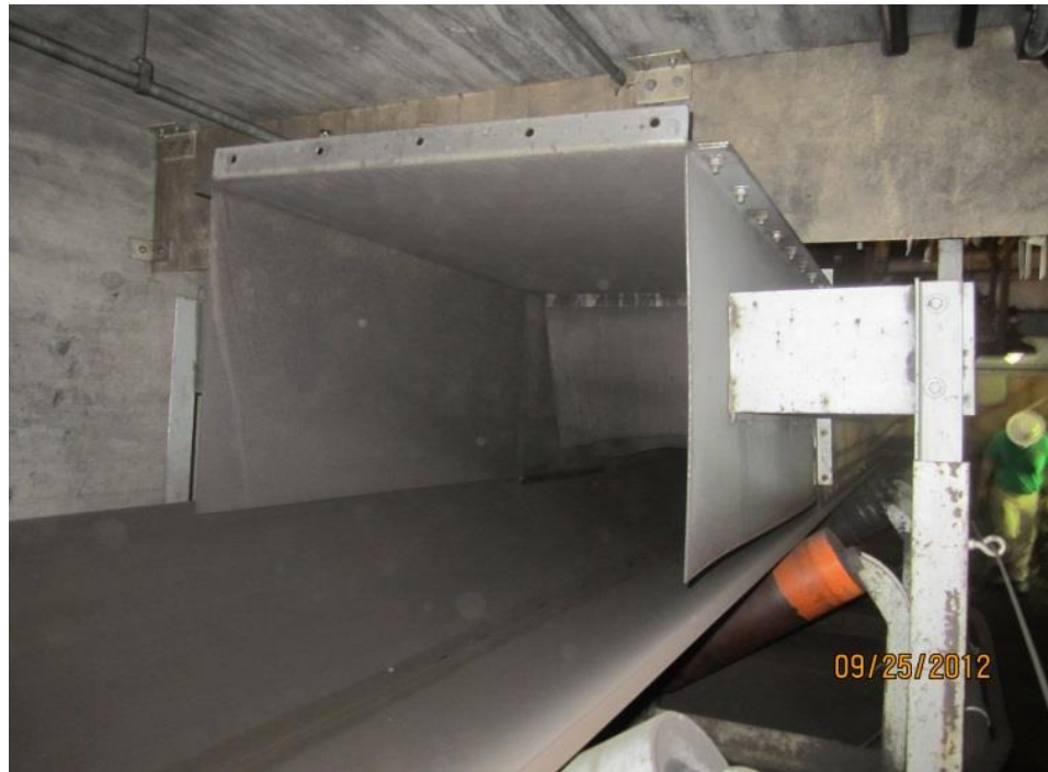
Picture 9: A skirt box too wide as observed at BRF on September 25, 2012, along BC-7. Skirt boxes that are too wide cause coal leaks.
