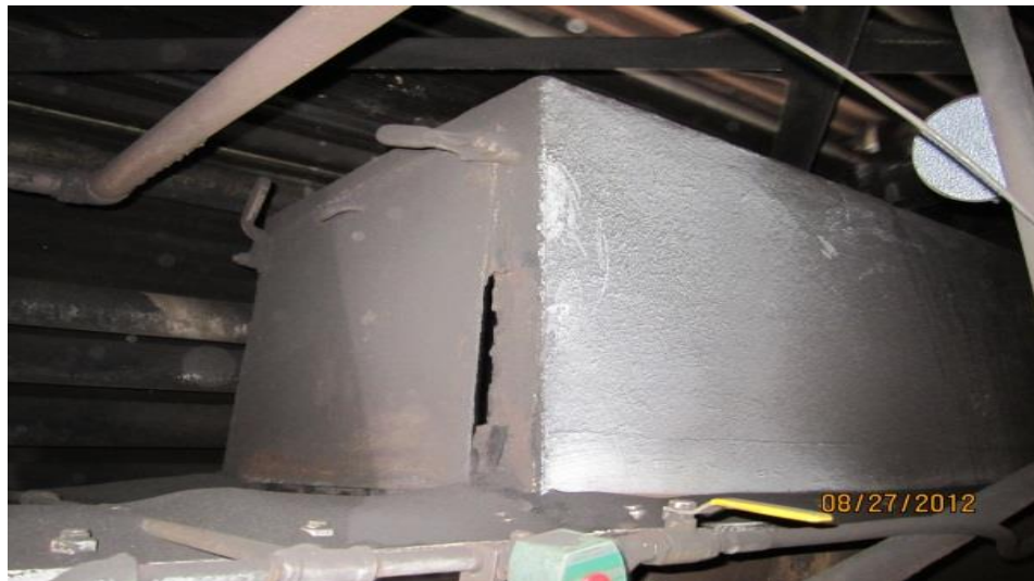
Picture 5: Deterioration around the skirt box opening allowing coal dust to escape as observed at PAF on August 27, 2012, in the West Bunker room.
