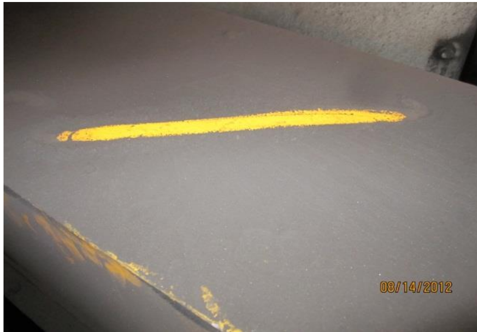
Picture 1: Dust accumulations greater than 1/32 inch, as observed during our walkdown at CUF on August 14, 2012. This is a beam on top of the Surge Hopper building.
