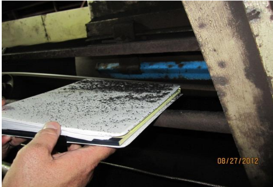
Picture 6: A skirting system in need of adjustment or replacement as observed at PAF on August 27, 2012, in the West Bunker room (BC-22). Misaligned skirts cause coal dust leaks. This picture illustrates coal leaking onto a white notebook held by the Auditor.
