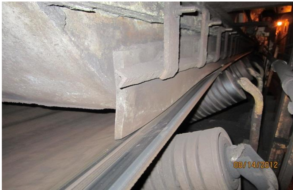
Picture 7: A skirt seal in need of alignment as observed at CUF on August 14, 2012, in Silo 1 (BC-9).
