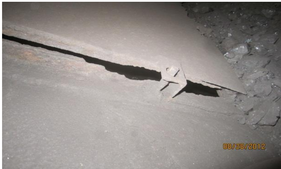
Picture 3: A deteriorated seal around the chute door as observed at PAF on August 28, 2012, located at the Alpha Station Breaker. Deterioration in the chute allows coal dust to escape.
