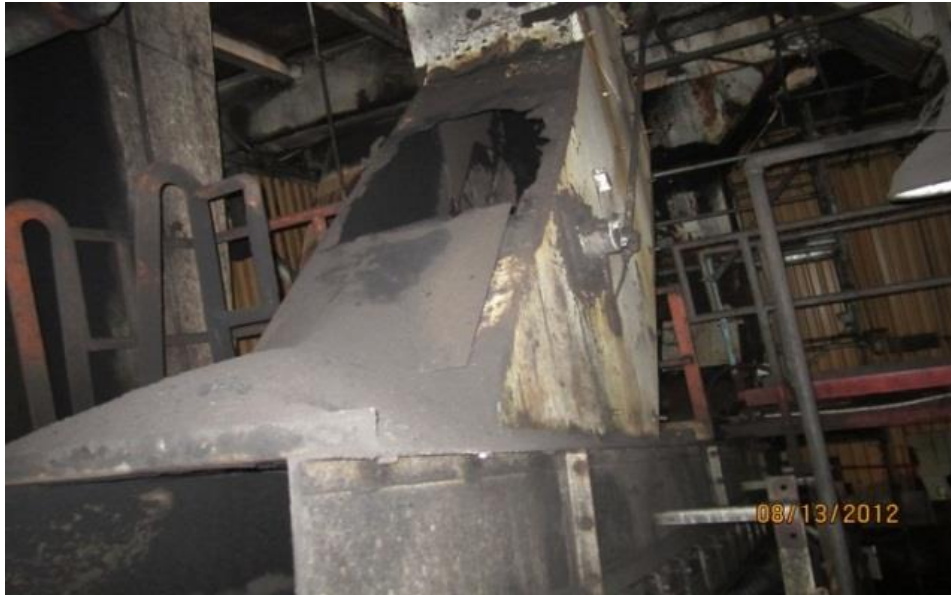
Picture 4: A deteriorated chute allowing coal dust to escape as observed at CUF on August 13, 2012, located at Transfer Station B.
