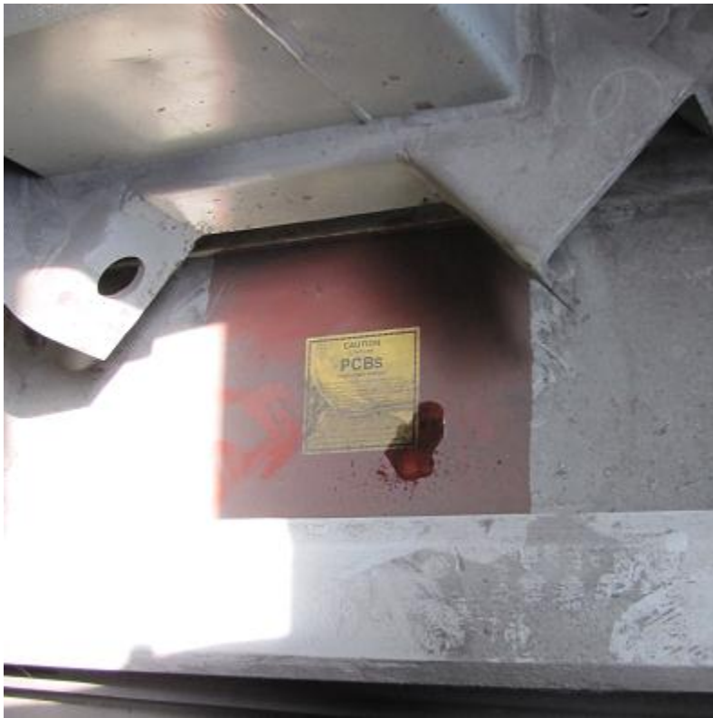
Figure 9: Spill From Leaking PCB Equipment
