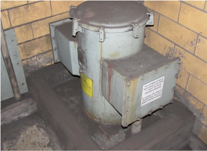
Figure 6: PCB Equipment Covered in Coal Dust
