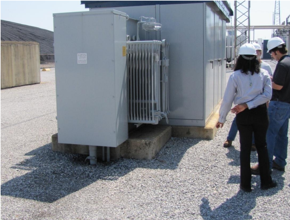
Figure 8: PCB Transformer Lacking Containment Dikes
