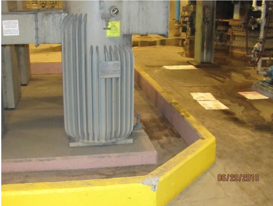
Figure 7: Cleanup Rags Within Five Meters of PCB Transformer
