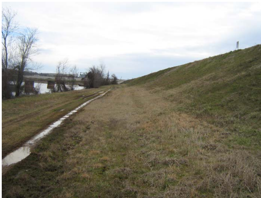
Photo 4 Northeast Dike prior to remedial construction.
